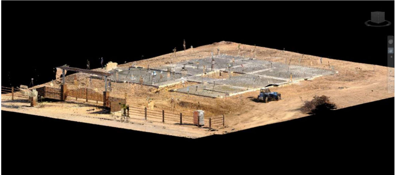
Figure 11: This is a portion of the FARO S150 data for the slab on grade. The pristine condition of the slab was great for capturing clean content, but also made it difficult to register due to a lack of reference objects.
